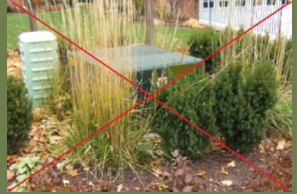
Obstruction around a transformer
