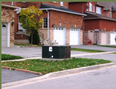
Pad mounted transformer
