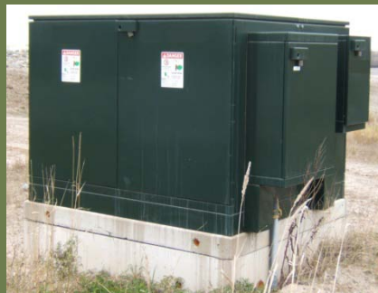
Pad mounted switchgear
