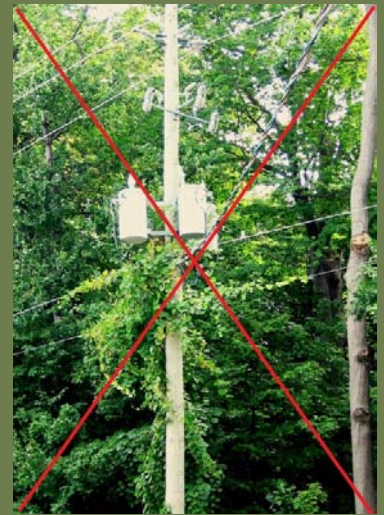
Pole growth contacting electrical equipment & powerlines
